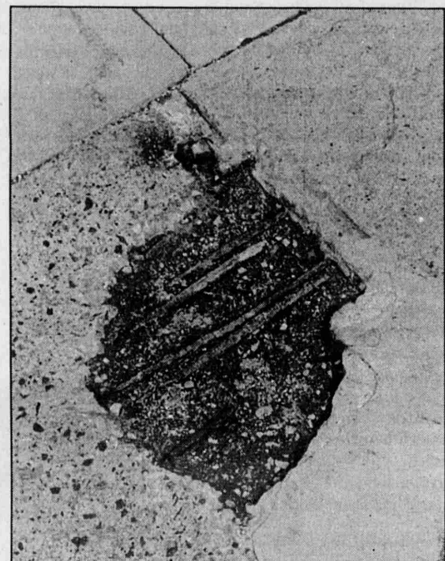
This dent in the sidewalk along the Main Street bridge is among several the Michigan Department of Transportation plans to repair this week. The work will be done in time for the start of the Riverwalk Festival, July 7-10 in downtown Lowell.
