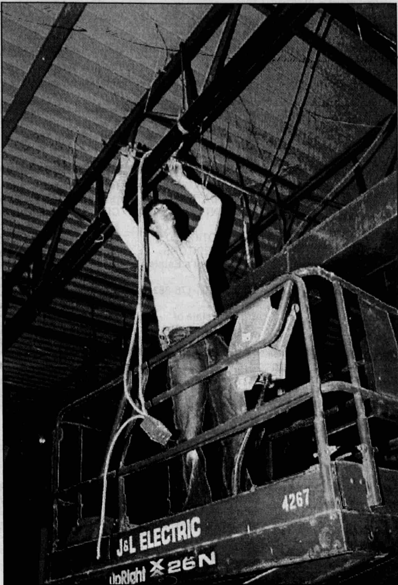
Mike Hamilton, an electrician with J&L Electric of Battle Creek, is shown removing wiring from the former Family Fare grocery. Construction began last week to get the space ready for Tractor Supply Company store. The store should open in mid-May.
