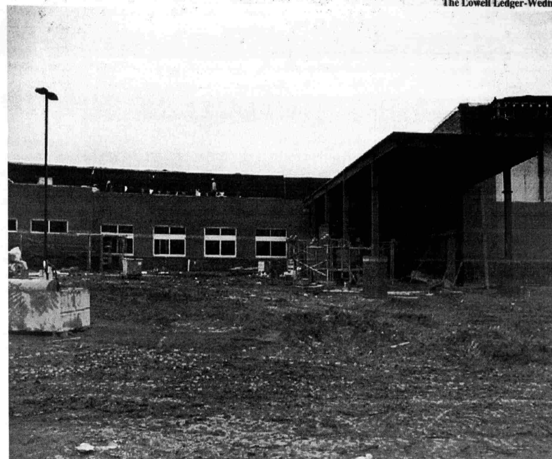
By early December, the exterior brickwork was complete at the new Murray Lake Elementary. There will be an open house at the new school building Sat., Jan. 17 from 1 to 3 p.m.
