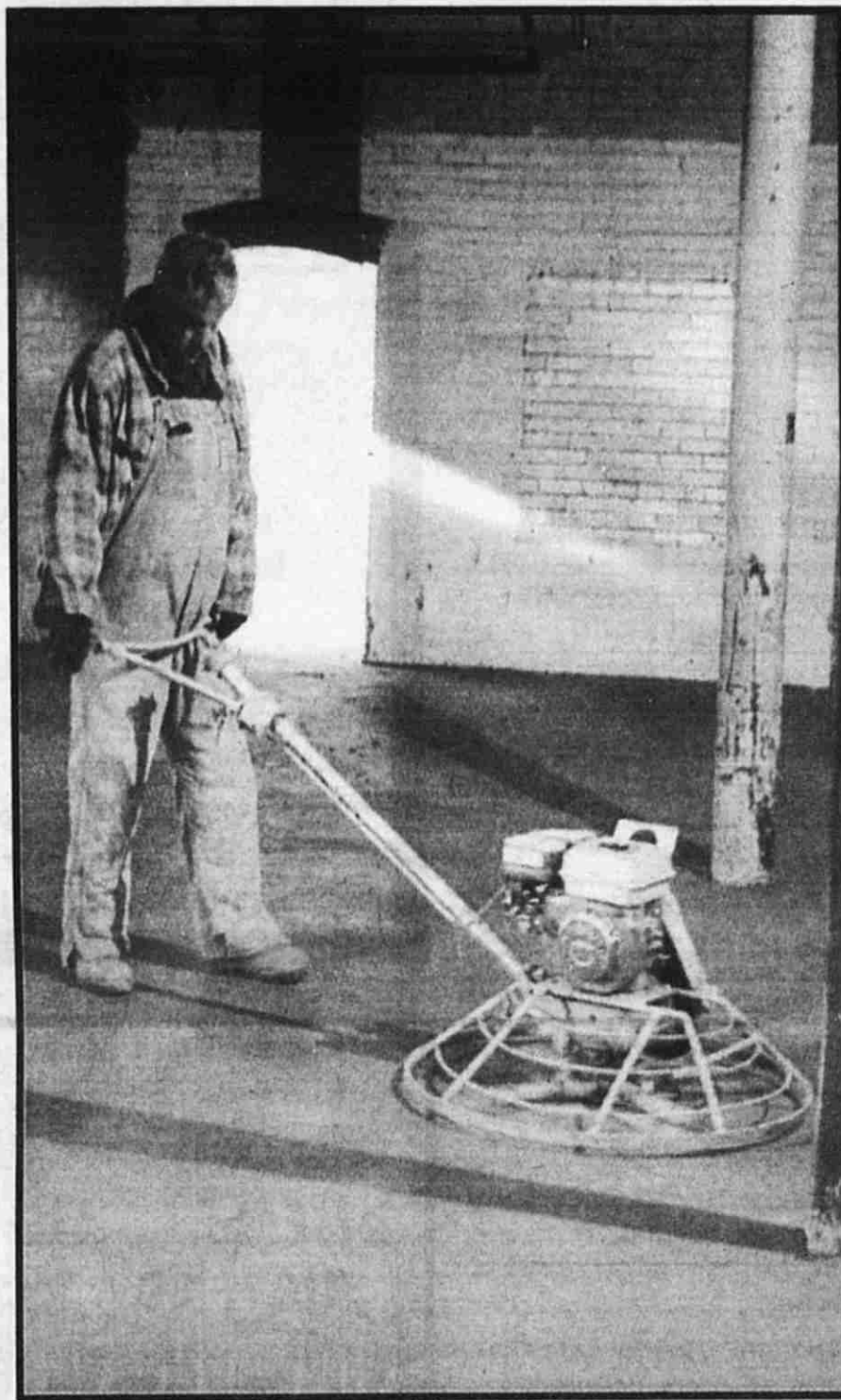
Marc Casemier, of Davis Construction, in Grand Rapids, works to smooth the cement floor poured in City Hall.
