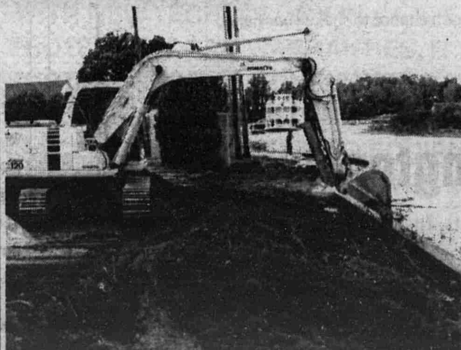
Work to extend the Riverwalk along Flat River continues into week three. Above the new boat landing dock can be seen. Right, machinery can be seen clearing brush.
