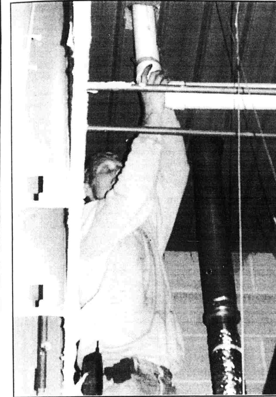
Jeff Brown, Canfield Heating and Plumbing, works at the YMCA fitness center.
