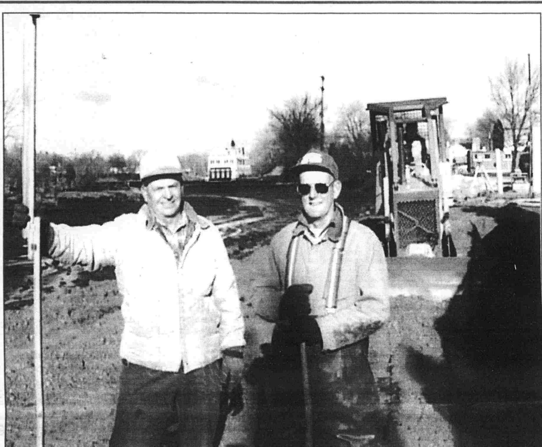
Rich Bieri, left, of Bieri & Sons Excavating, and Ivan Blough worked with Joel Bieri Monday to level off the sloped bottom of the Flat River in front of the boat launch.
