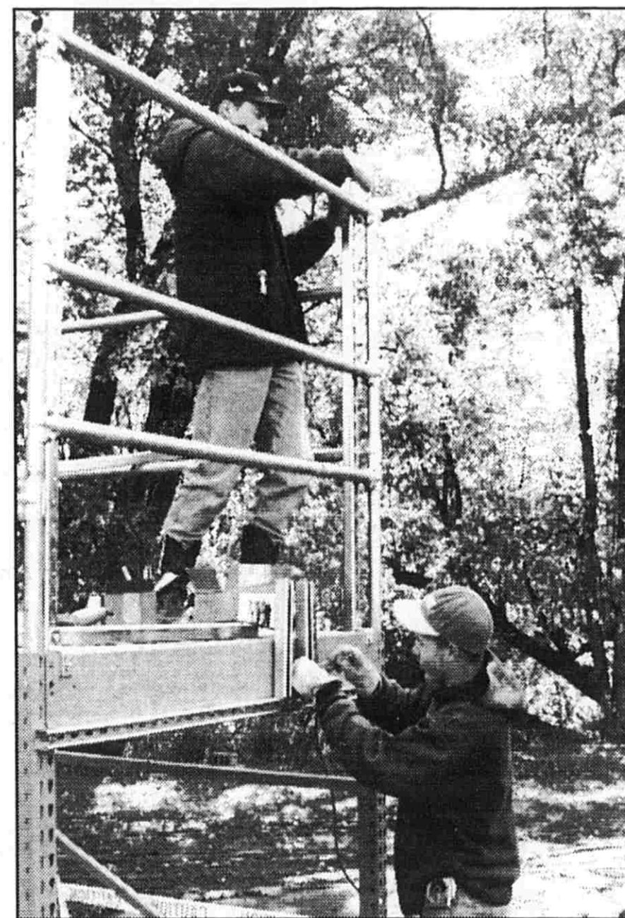
Mike VanTimmeren, left, and Ken VanSpronsen, of Associated Electric, completed the electrical hookup on Wednesday.
