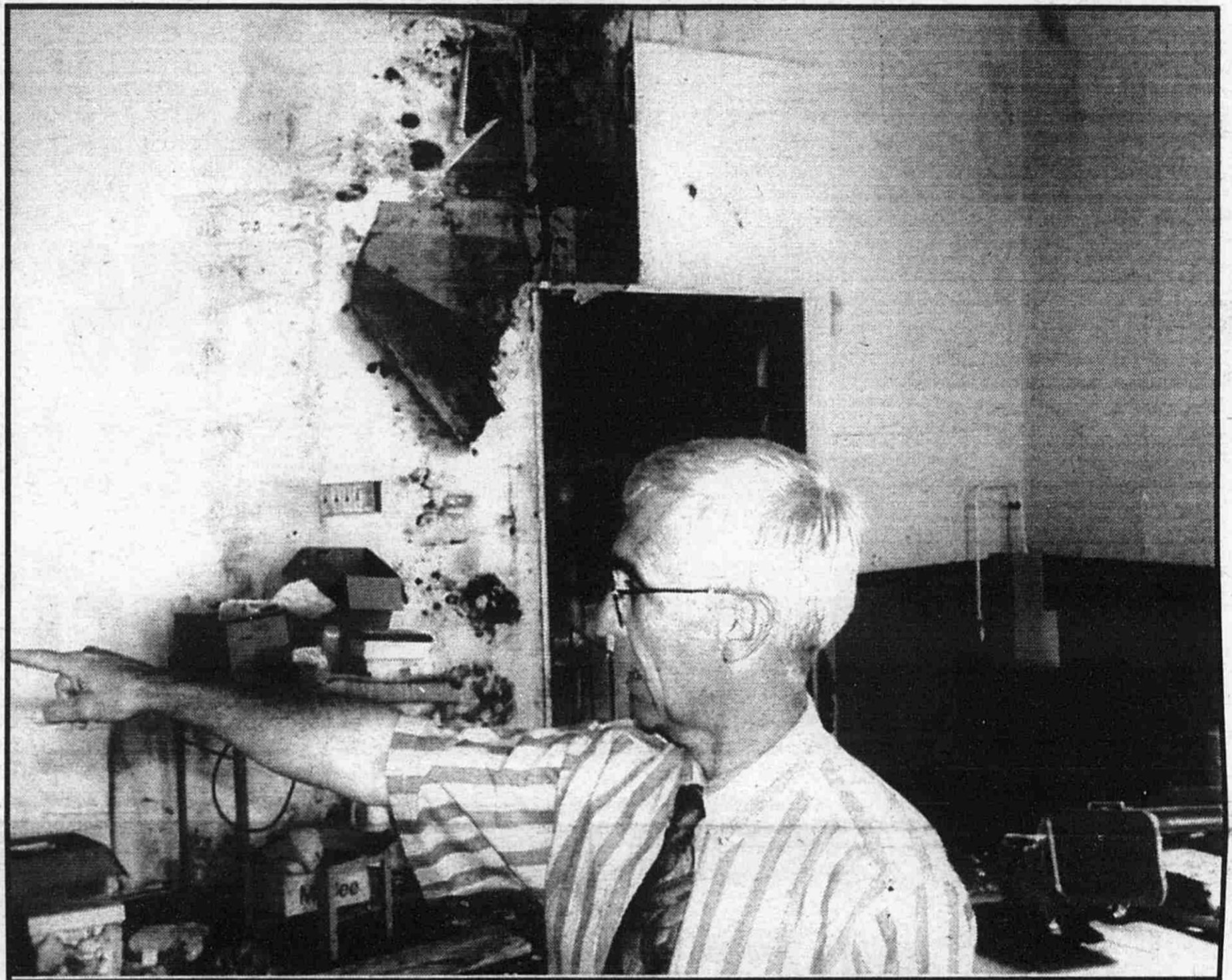
First Congregational Church pastor Roger LaWarre identifies areas of the old Baptist Church in need of repair.
