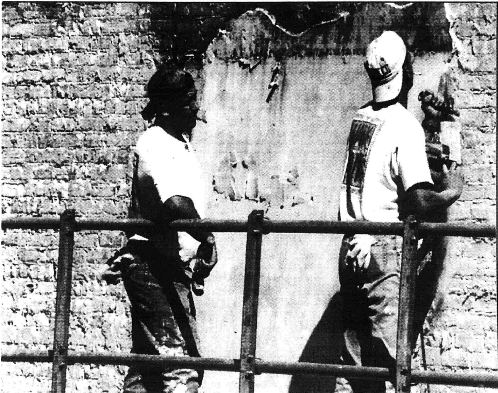
Architectural Building Restoration, Inc., 2775 Tyler Trail employees, Tim Koetje (left) and Lou Pelagio, remove the sheets of plaster from the outer wall of the Lowell Serenity Club. Pelagio operates an electric chipping hammer to dislodge the plaster from the brick. To help loosen the bond between the plaster and brick, the plaster is hit with a blunt hammer before the chipping instrument is used. Mark Batchelor, sales manager/owner of the company, will fill the joist pockets, remove as much of the tar from the brick as possible and reset four to five courses of brick before winter sets in. In the spring, the company will remove isolated spots of plaster from the wall and then seal the brick with a color sealer. The Lowell company is a historical building preservation specialist. Batchelor said he would provide any business in the downtown area with a free estimate on restoration of their brick buildings.
