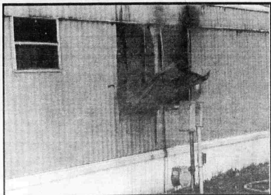
Damage was estimated at approximately $50,000. The trailer and items inside were destroyed.
