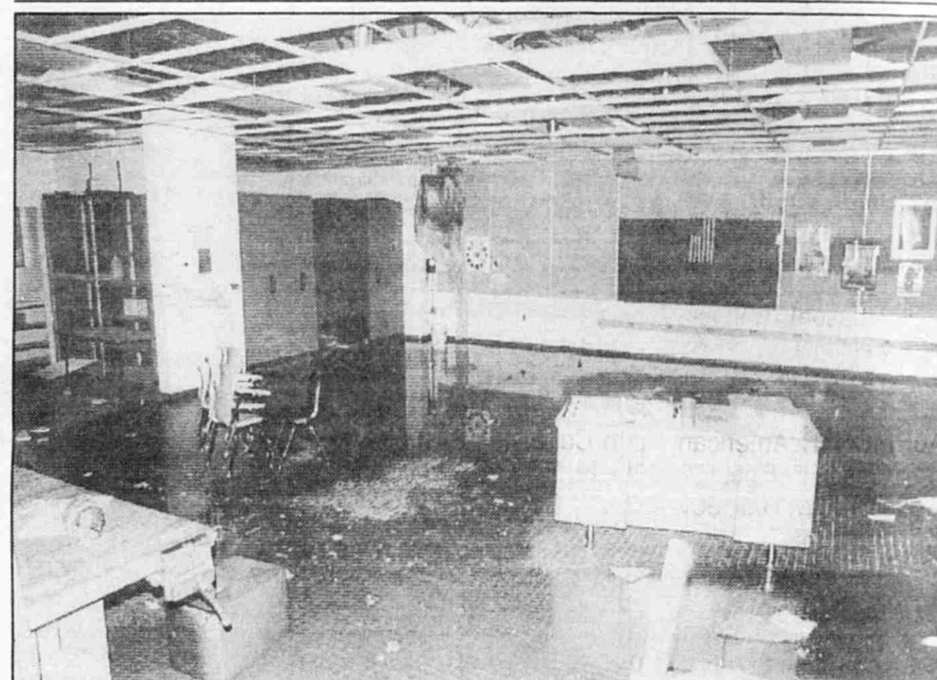
Ceiling and floor tile were casualties of the roof leak at Cherry Creek Elementary.
