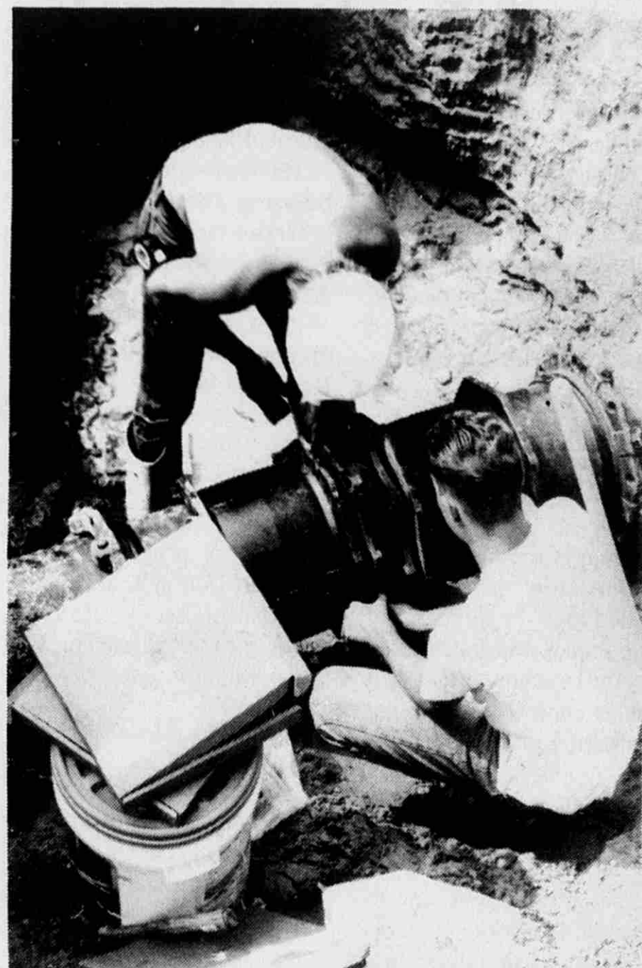
Bill Hoye, left, and Matt Roach from Jen-Kel Construction, Grandville, make the final connection joining Lowell Township and Lowell School water mains.
