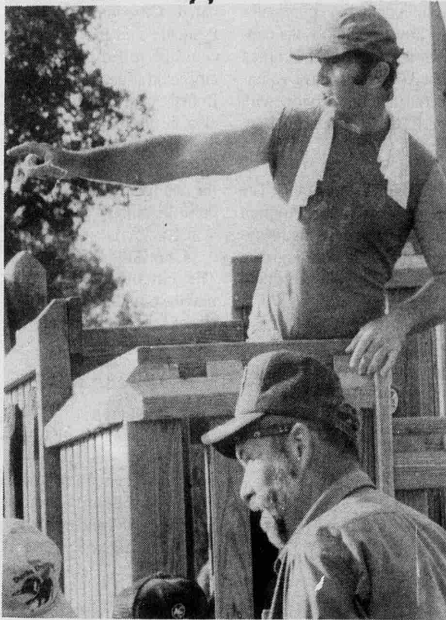
Creekside Kingdom construction consultant Mike Finn points while giving instructions to Lowell's Dean Lonick.
