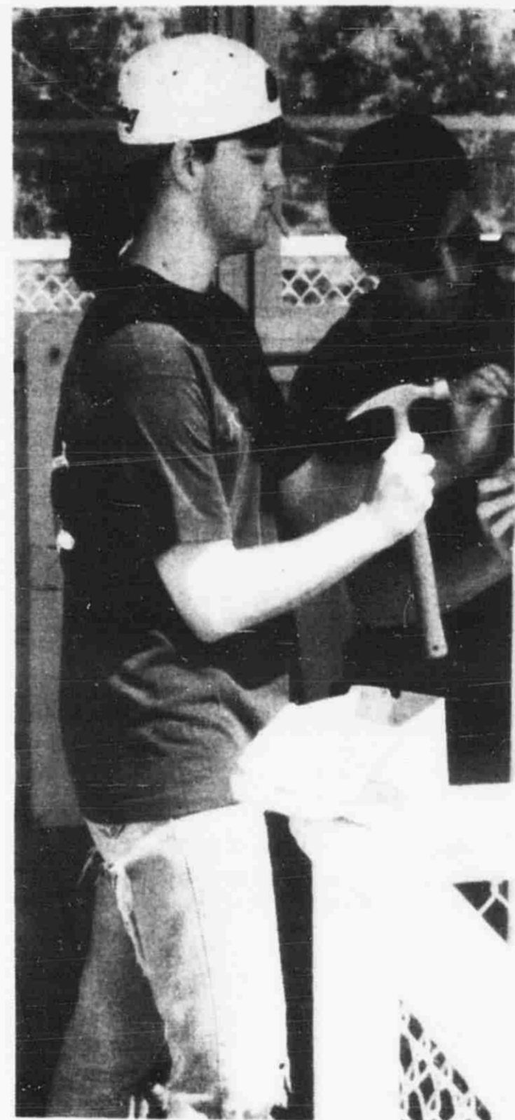
Lowell High School students took the time to repair damage to the Showboat inflicted by vandals. The day work insured graduation at the Lowell Showboat.
