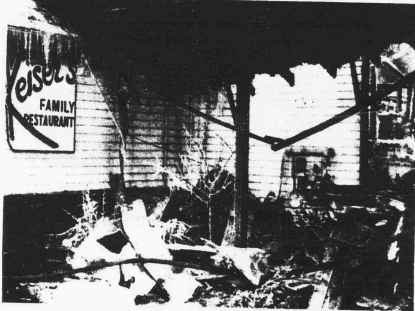
The morning after, showed the aftermath, of a fire that destroyed the building of Lowell's oldest merchant. The state fire marshal report stated that the cause of the blaze at Keiser's Kitchen was electrical.
