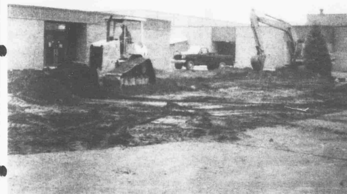
Renovation work on the high school has begun on the west end. The plans call for the high school to be turned into a middle school.
