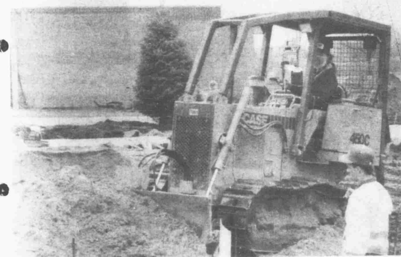
Moving ground in preparation for renovation work on the west end of the high school.
