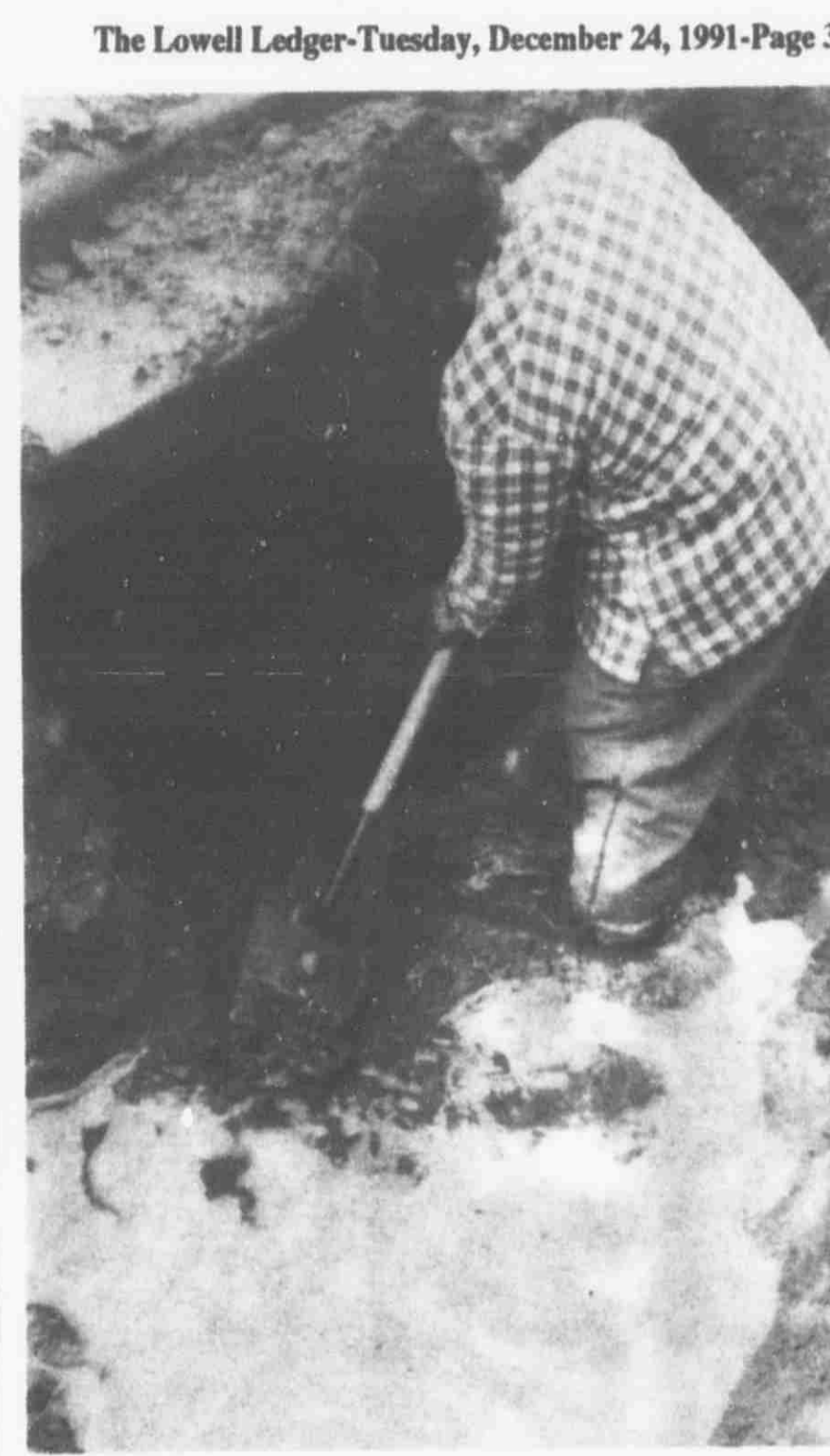
A broken water main was cause for some November pipe repair on Hudson Street.
