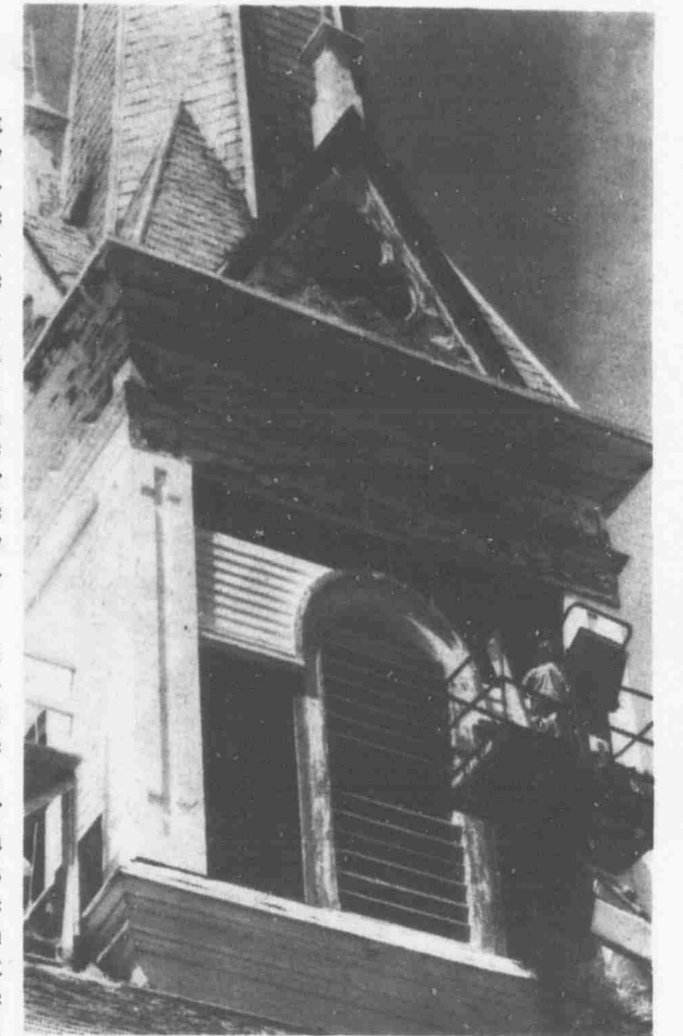
A $300,000 renovation project, was started on St. Patrick's Catholic Church in Parnell.
