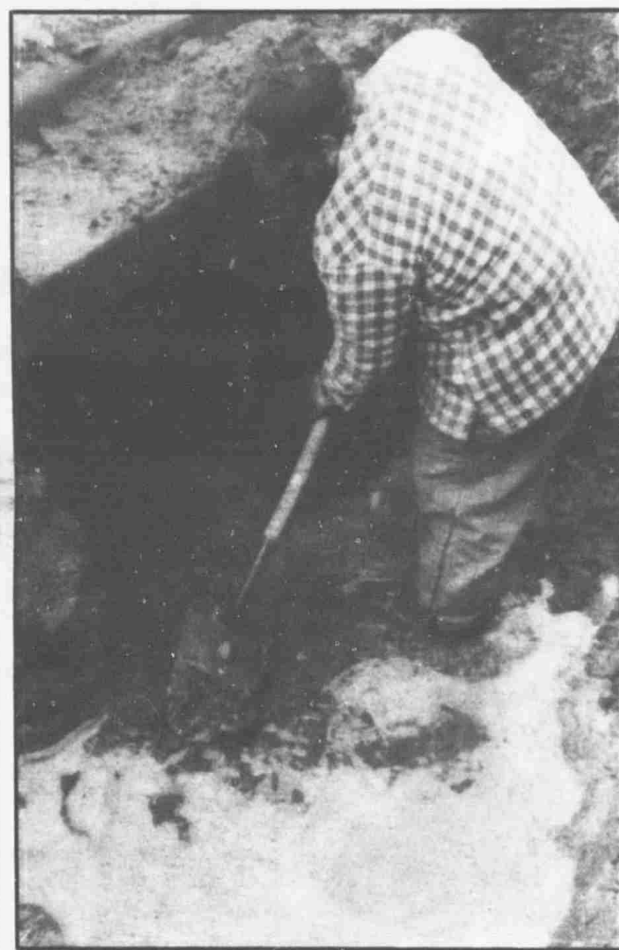
A broken water main north of town on Hudson Street, kept Lowell Department of Public Works busy Monday morning.
