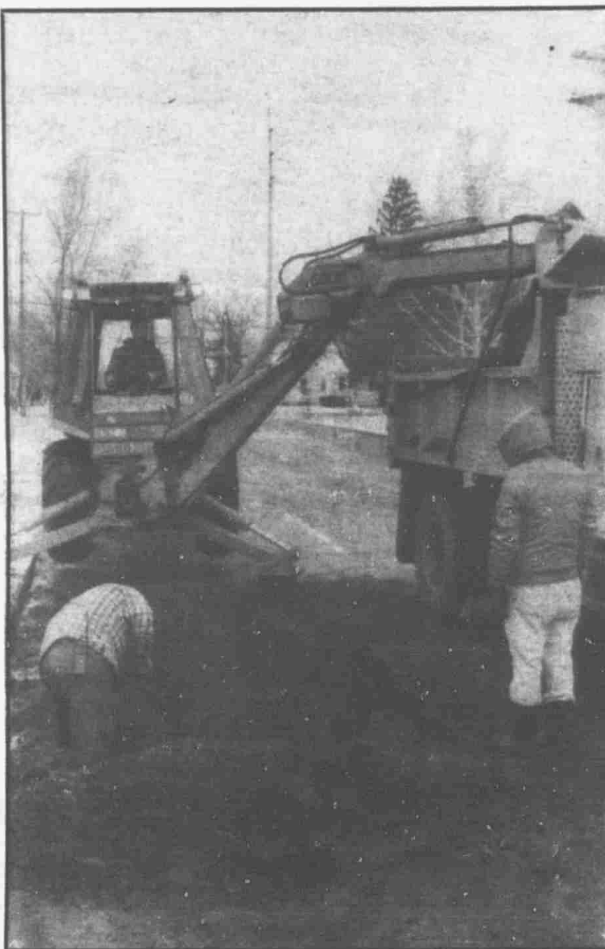
A broken water main was top priority Monday morning.
