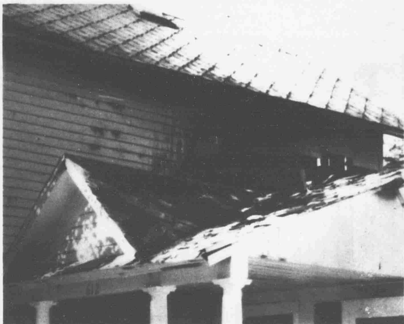
Lowell Fire Chief Frank Martin estimated the damage to the Melton home to be at $60,000.
