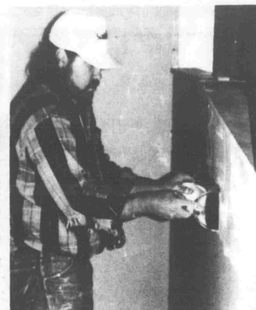
Brian Becker, foreman, Rapid Construction, works to complete the police station addition.
