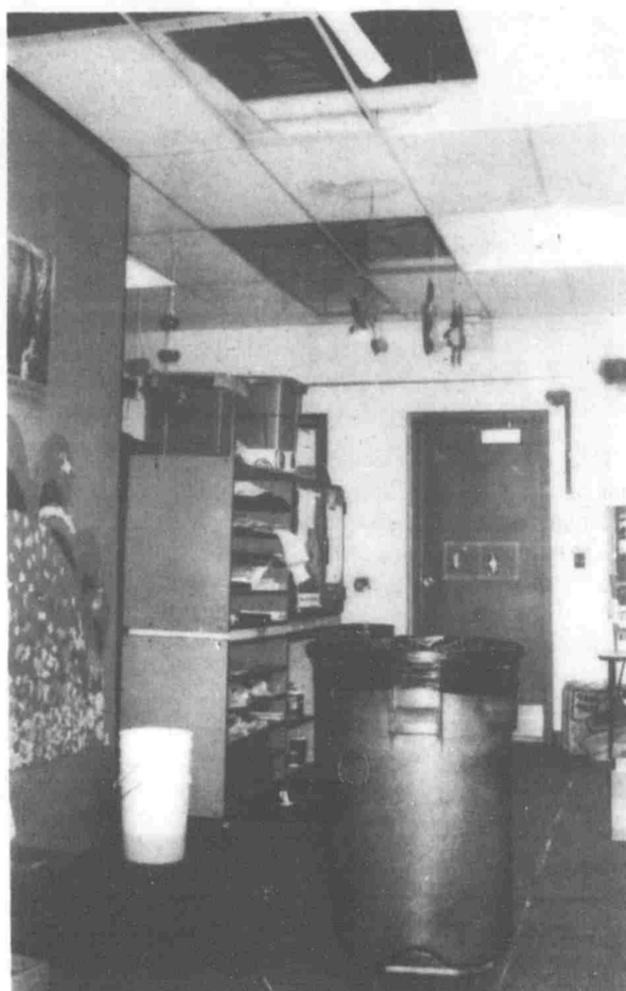
Troughs and plastic garbage cans are currently used to catch the water that comes from a leaky Bushnell roof. Bushnell is scheduled to be re-roofed this summer.
