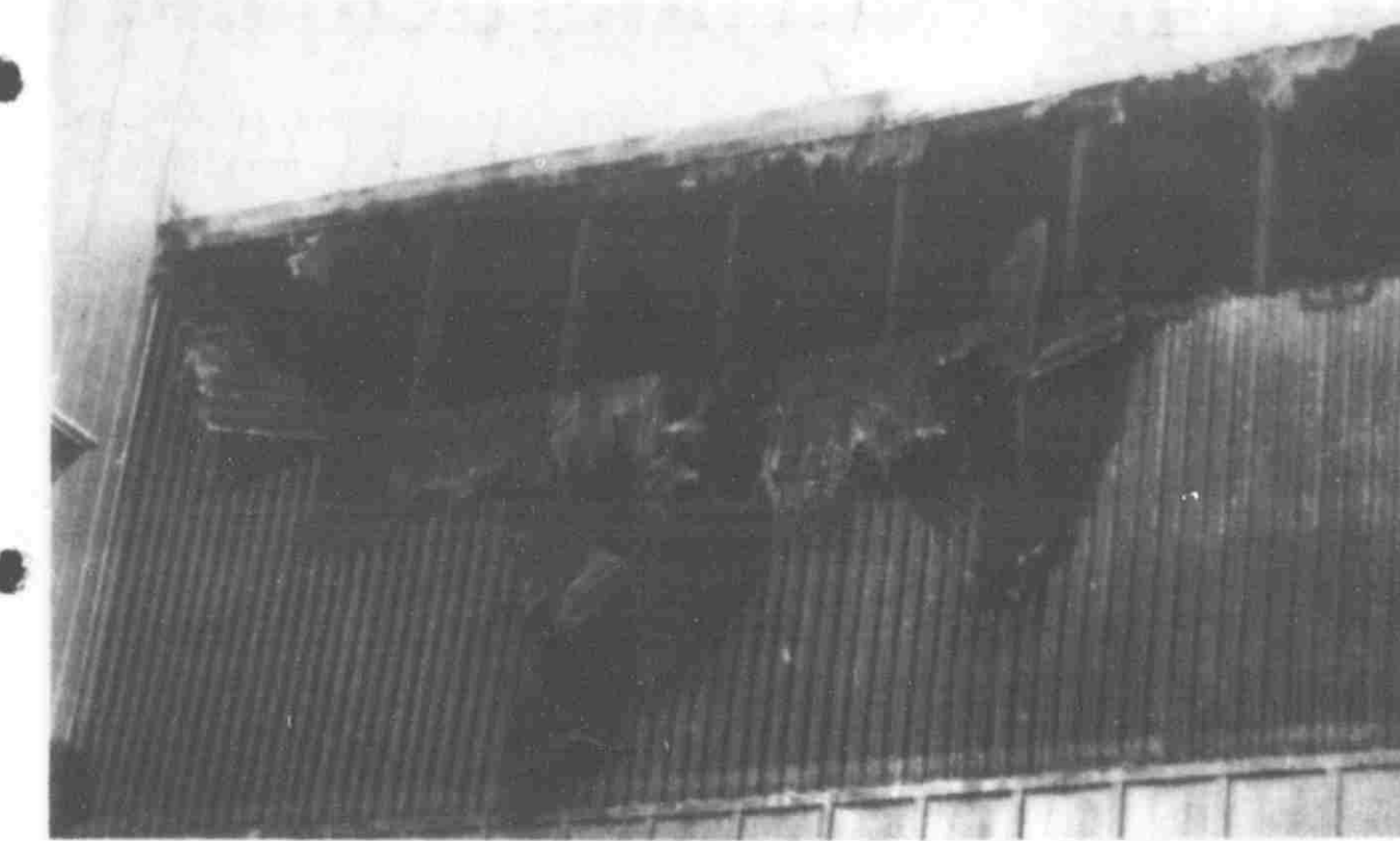
The plastic window above the tanks was destroyed.
