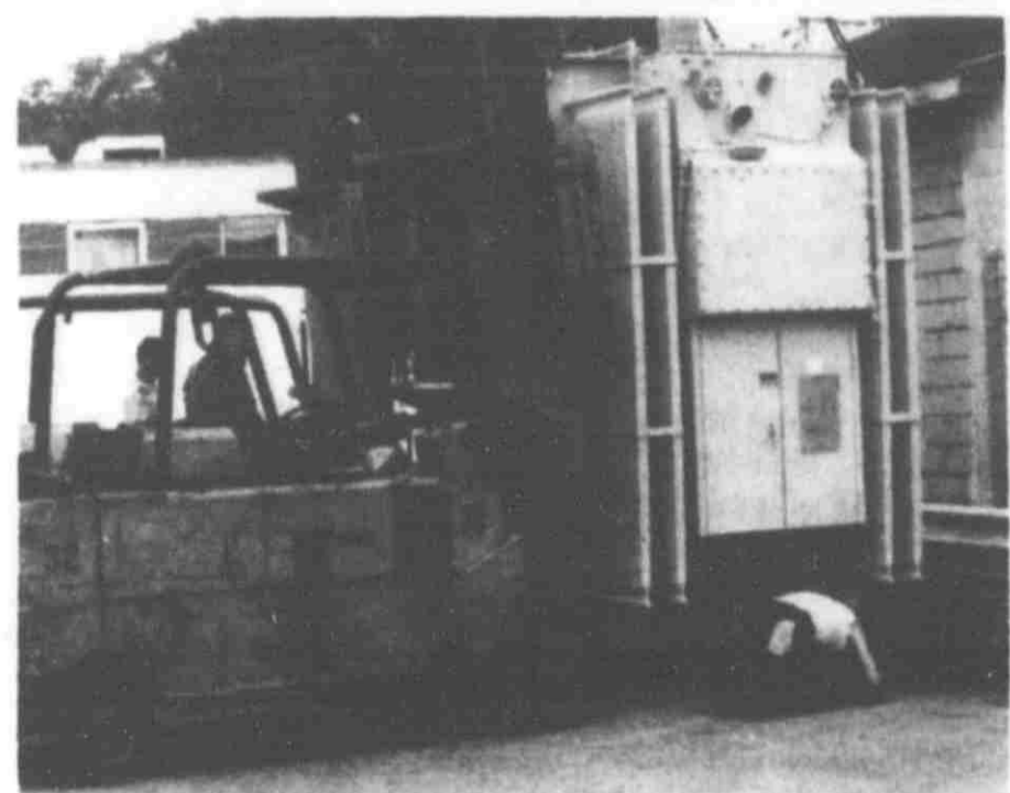
This is one of two hi-los needed to lift the transformer off of the flatbed truck.
