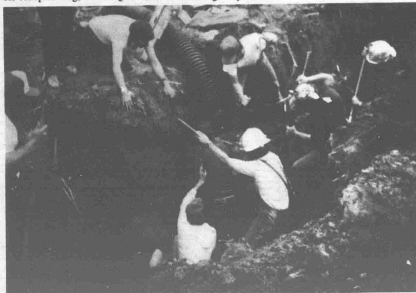
Rescue Units and paramedics worked for approximately an hour, freeing Don Bergy from the soil that covered him, after the walls of a trench that was being dug for a field tile collapsed on him.
