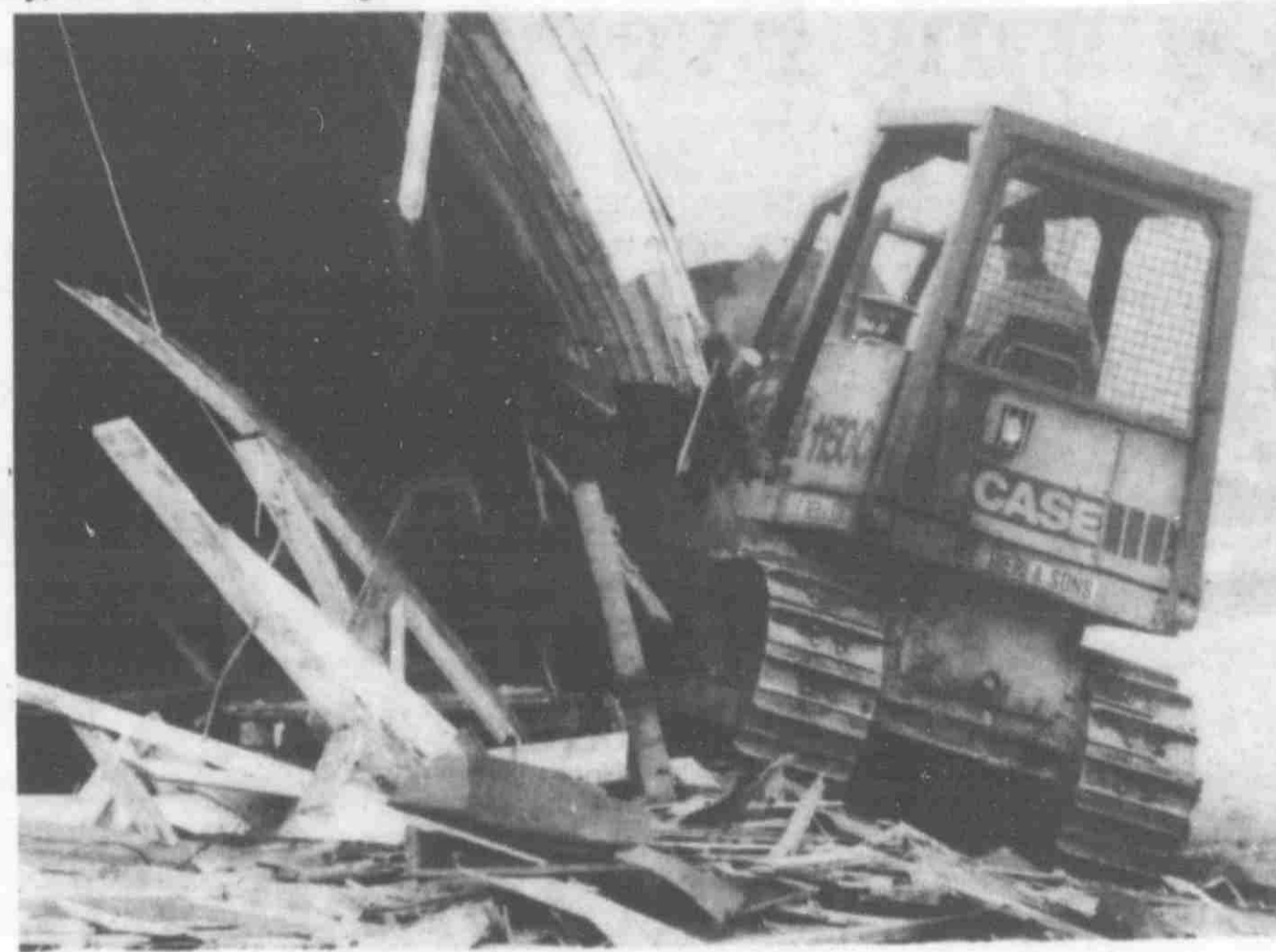
The Quanset Hut made from bent wood was knocked down by O.E. Bieri & Sons Construction.
