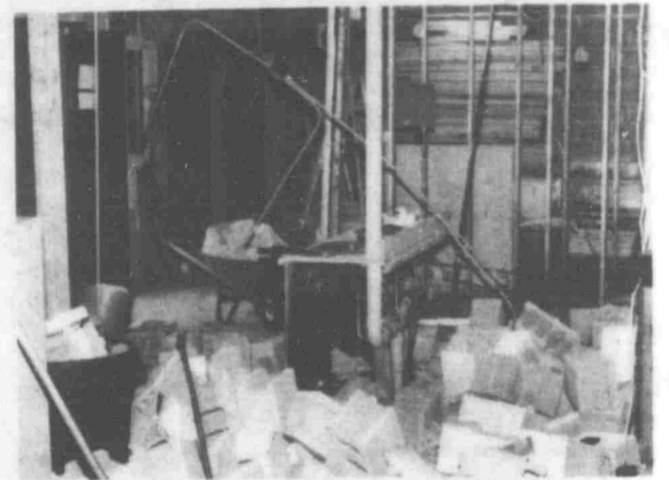
Renovations are underway at the former Paul's Showboat Restaurant. If work is completed on time, Keiser's Kitchen is scheduled to open its doors at the location come May.
