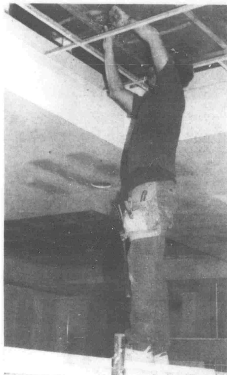
An employee of Dan Vos Construction helps do his part in getting Dari's Restaurant and Banquet Hall ready for its February opening.
