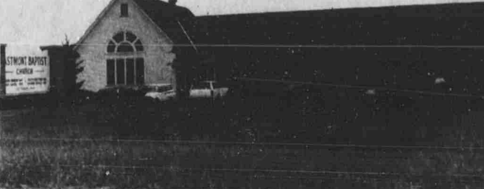
NEW ADDITION to Eastmont Baptist Church is nearing completion. Membership in the church has doubled in the last three years, necessitating the new structure.
