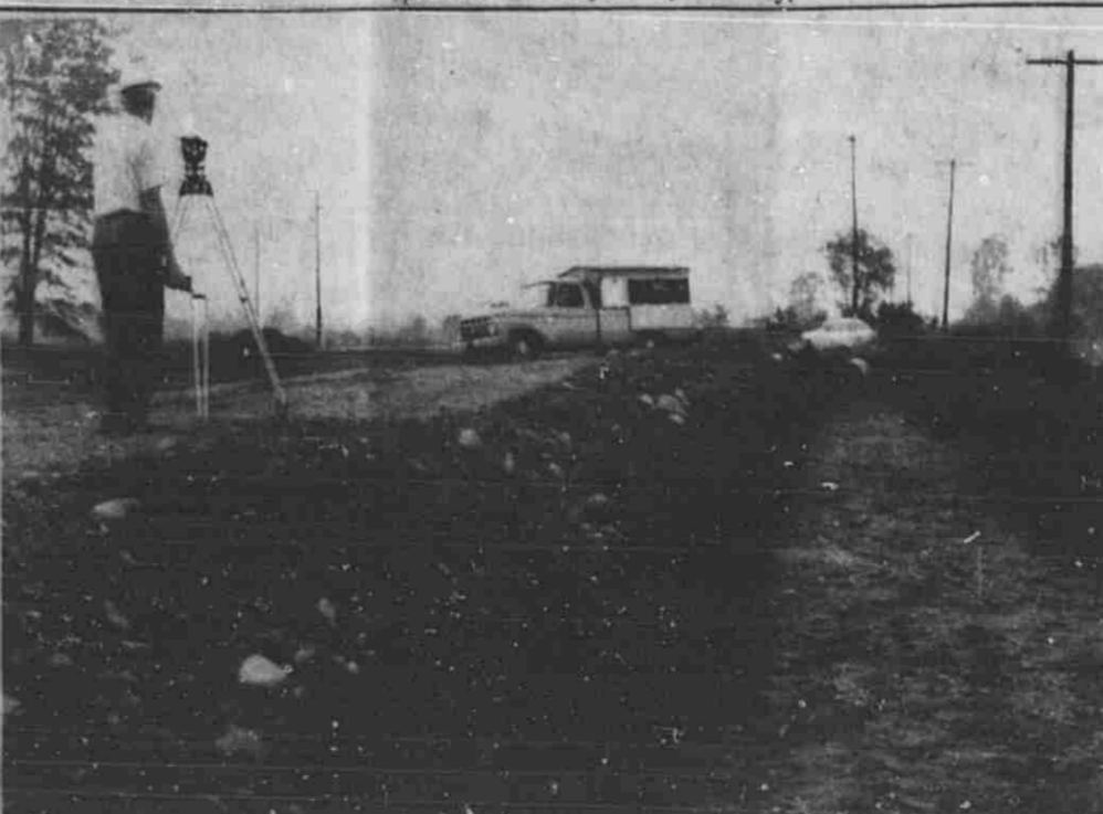
START OF CONSTRUCTION on the new Root-Lowell plant in northwest Lowell is underway with the initial phase of the project shown above. Footings for the walls will be poured soon. The plant and new equipment, a $ million project, is scheduled for completion in early December.
