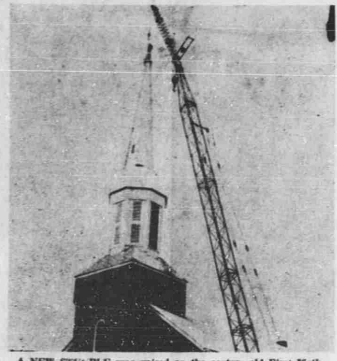
A NEW STEEPLE was raised on the century-old First Methodist Church of Lowell Monday. The church had been without a steeple since the early 1940's, according to Reverend Robert G. Weber. Plans to add the steeple had been initiated by Gougl Rivette, former chairman of trustees, and completed under the supervision of his successor, Stanley Gardner. Designed by Jon Walter of Lowell and constructed by Bieri Bros. of Lowell, the steeple was raised in place by DeVries & Sons of Grand Rapids.
