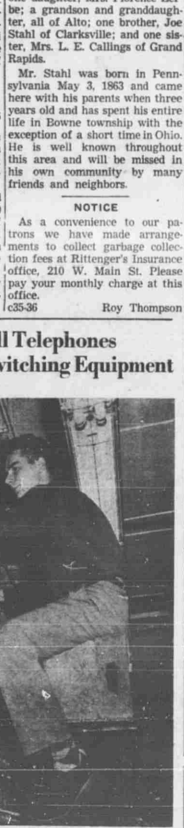
Robert C. O'Neill, Western Electric Company installer, is shown making one of the thousands of hand-soldered connections necessary to tie Lowell telephones into the dial switching equipment in the new central office building on Hudson Street.
