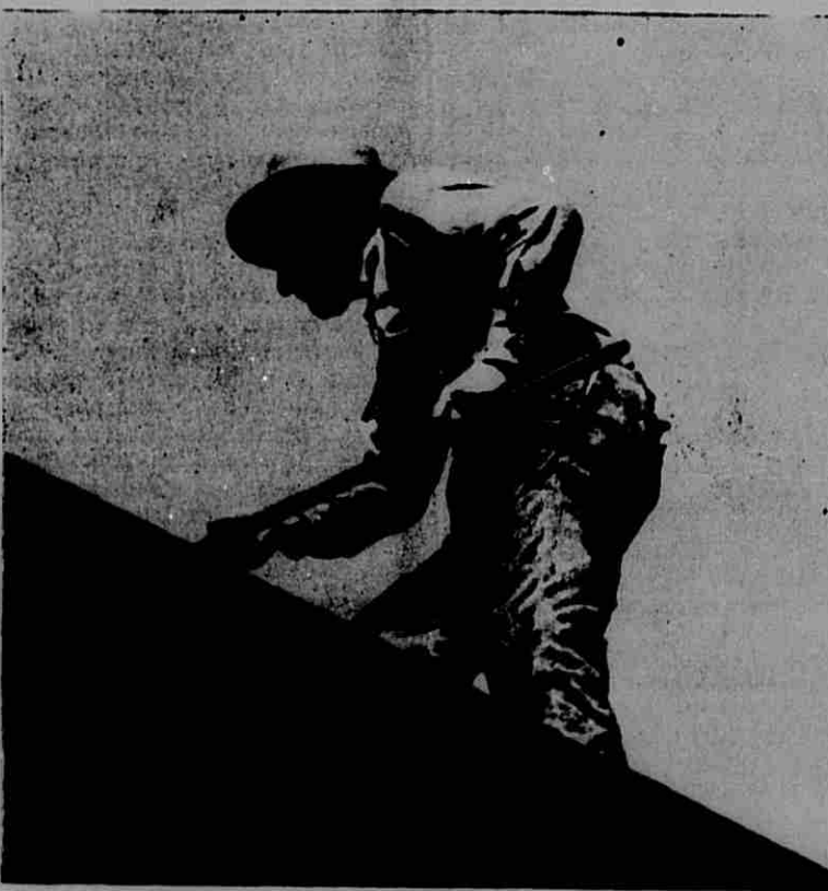
"Dick" Bergin, 90, will be surprised when he sees this picture. He was so busy at the time repairing the roof of his house that he never dreamed there was a Ledger photographer within 40 miles.
