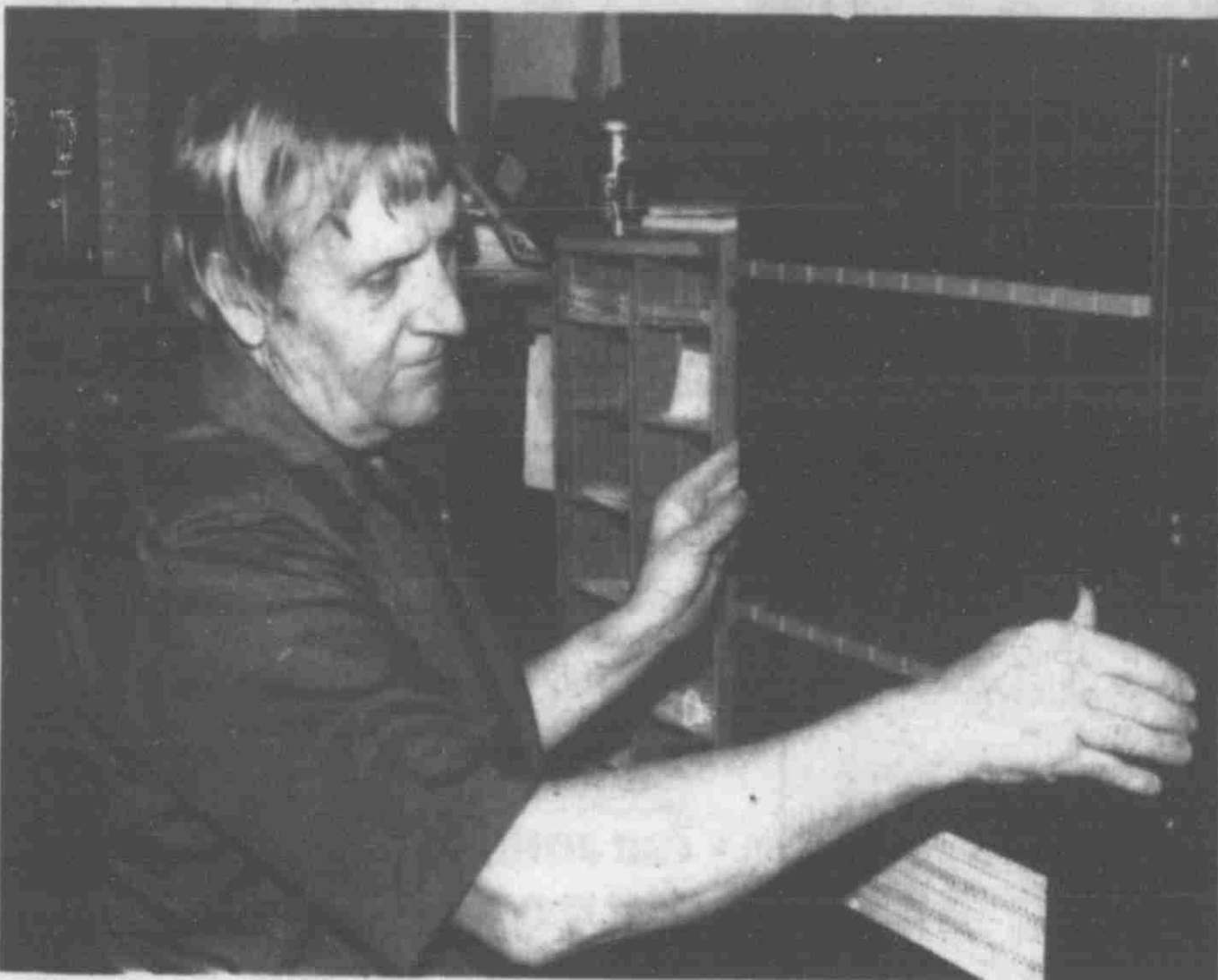
Bob Canfield, a switching equipment technician at Lowell's Michigan Bell switching station displays some of the new equipment installed to provide touch tone service to the "897" exchange.
