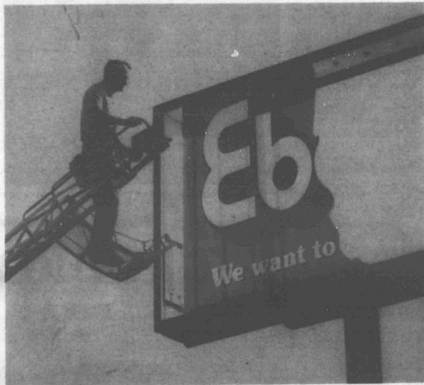
A workman on a boom truck works at removing what the storm left of Eberhard's lofty sign on Main Street. The sign was the least of their worries however, as the high winds created havoc with the store as it tore much of the roof allowing the rains to damage inventory inside.
