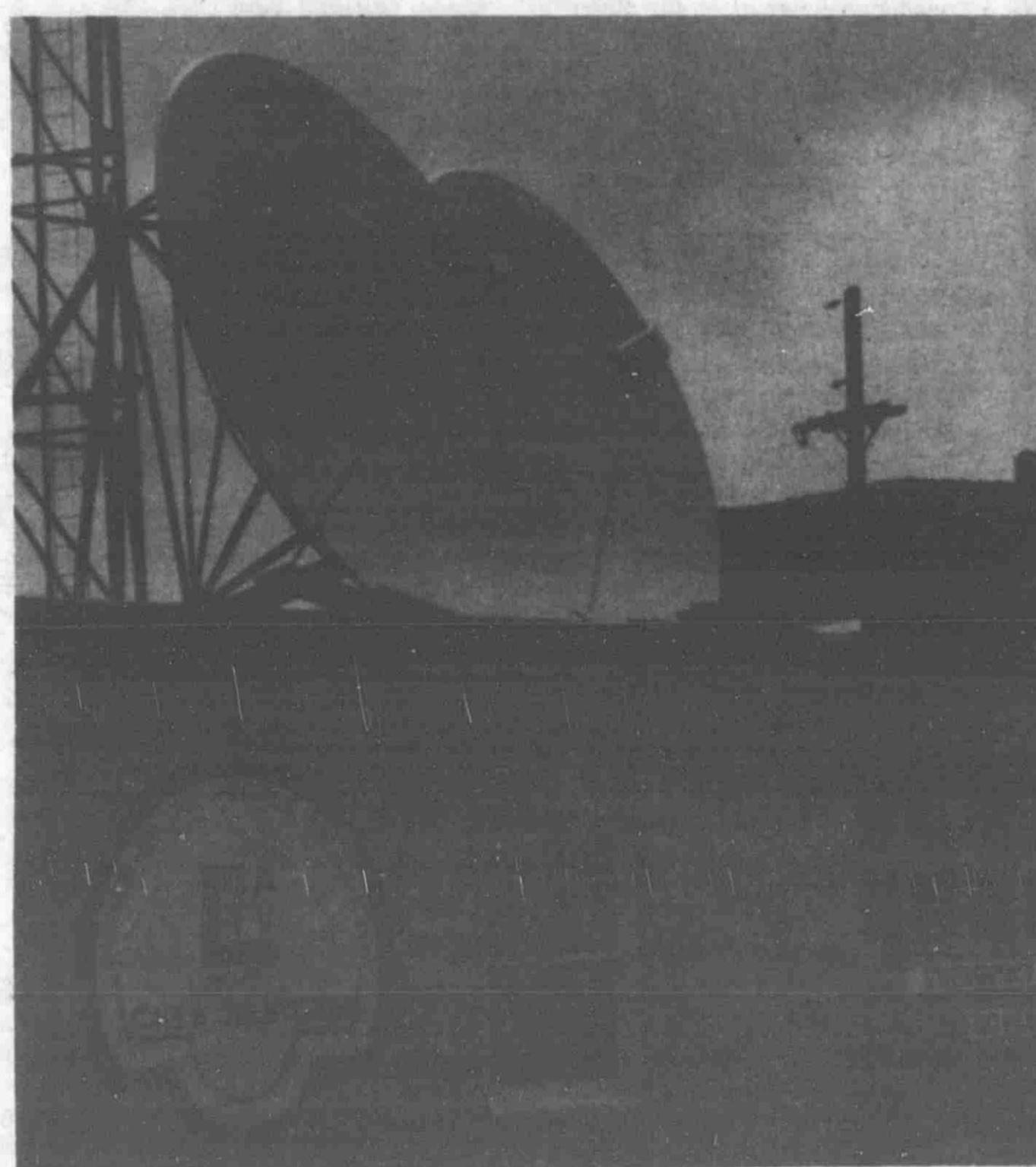
No... you're not seeing double. The Lowell Cable Television Department had to install another satellite receiving dish when Home Box Office switched their signal over to a different satellite. The new dish gives LCTV the option of picking up some other cable channels such as the Disney Channel.
