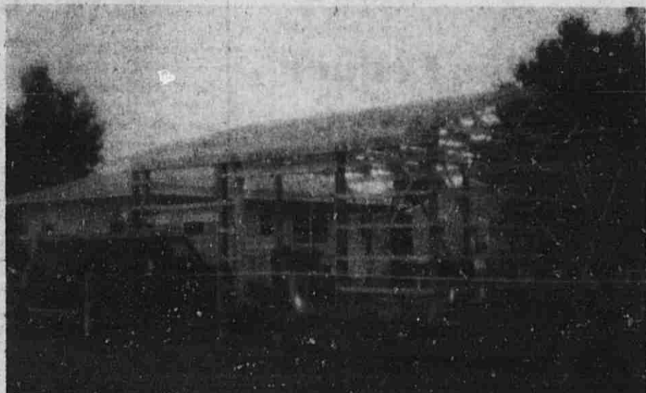
The roughed in structure belonging to Allen Hull will be lowered 4 feet, sided to match and attached to his residence to comply with a ruling set by the Lowell City Council.
