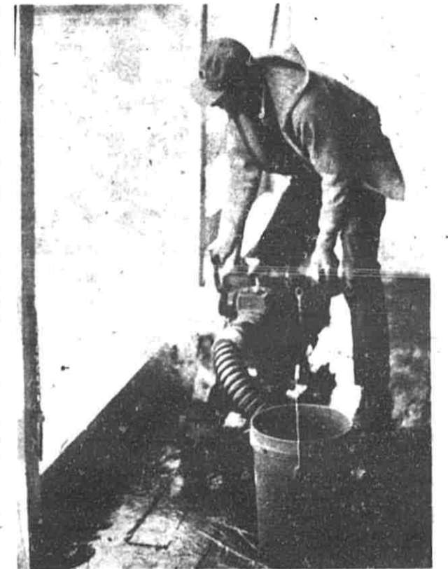
It looks like pumping the Spring run-off out of the pontoons which support the Lowell Showboat will be an annual event. Ivan Blough and a crew of workers manned the pumps on Tuesday and had the Robert E. Lee floating proudly once again. Blough is a member of the Showboat directors and built the boat in 1979.
