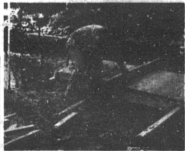
One of the bridge crew smooths the concrete capping on the east pier. The Thornapple River is in the background.—Photo by Dave Barnes.
