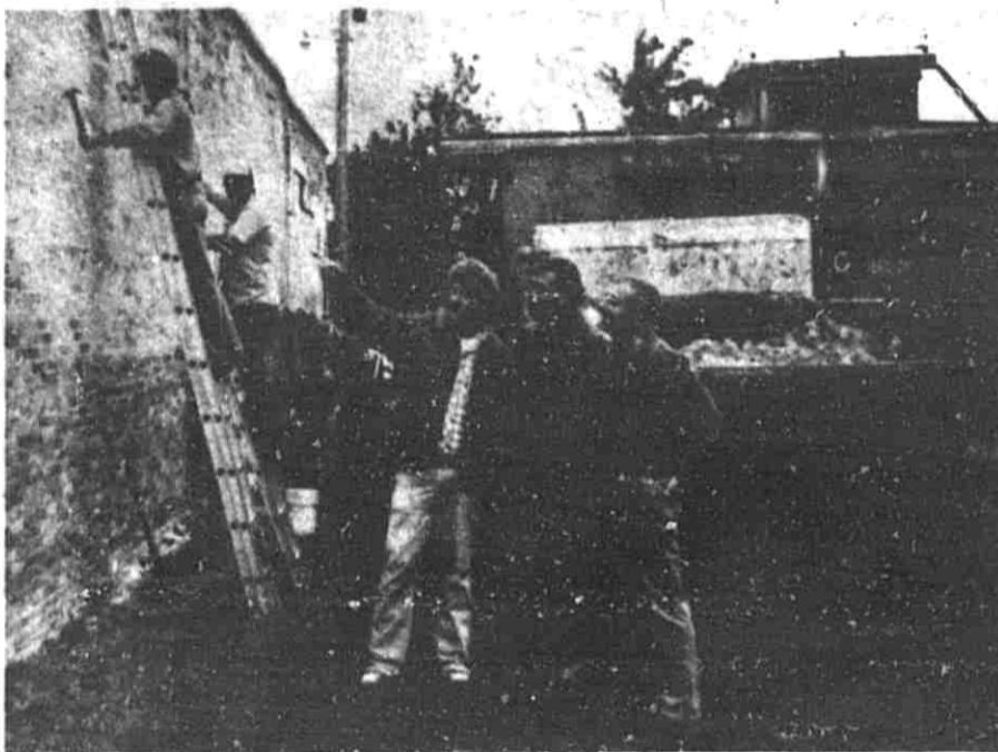
Kurt Albrecht, Lowell Area Jaycee Vice President and project chairman, Dean Collins, Mayor and Jim Hall, chairman of the Lowell Parks Commission observe volunteers removing old plaster from one of the buildings that border the new park. Murals will be painted on these walls in the future.
