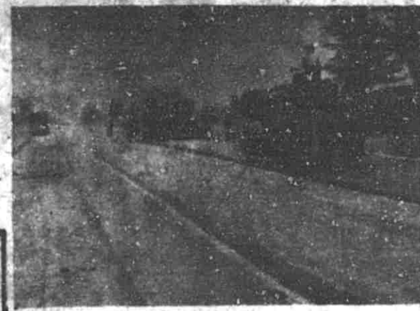
The large machines, background, lay and spread the blacktopping on the southbound lanes of M-37, followed by the compacting of the material by the roller.—Photo by Dave Barnes.
