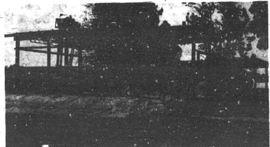
The steel superstructure of the new Department of Public Works and Fire Station #2 building on South Hudson and Ottawa Sts. is in place and work on the roof should be complete this week.
