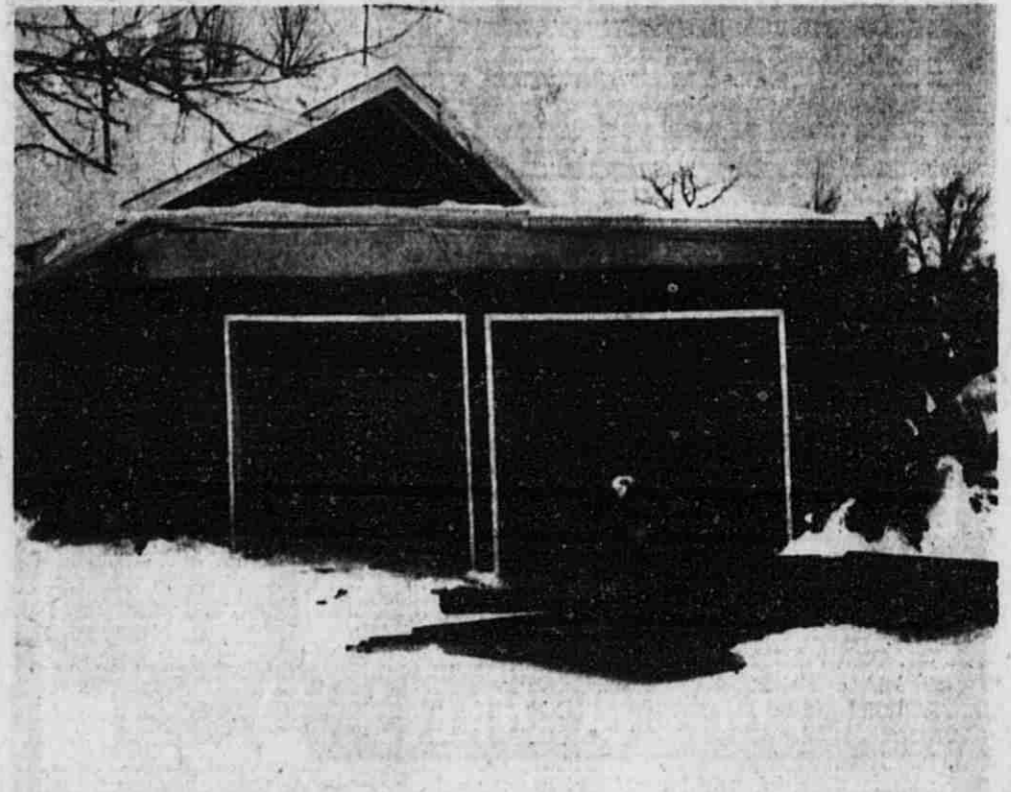
The Dennis Nead family in Saranac thought they heard a strange noise about 5 a.m. Sunday but couldn't see anything from their windows. Neighbors called about 8 a.m. to tell them that their two-stall garage had fallen in on top of their cars. The vehicles sustained moderate damage. Obviously, the garage is going to need some help.
