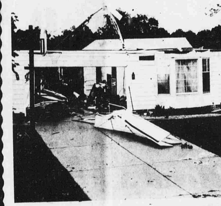
The residence of Mrs. Larry Biggs, Jr., 210 Wyandotte Ct., Saranac, had its entire roof removed and carried over 200 yards away. The home is in a subdivision but neighboring houses suffered no damage. Saranac had several trees and limbs downed by the storm but was not nearly so hard-hit as Lowell.
