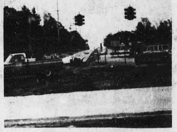
Two new lanes, center background, of M-21 will carry east and westbound traffic while the old two lanes, behind the barricades, will be removed and two new lanes for eastbound traffic are built.
