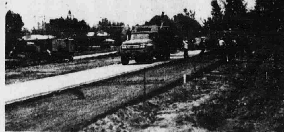
A crew positions the reinforcing steel prior to the pouring of concrete for another East Beltline lane looking south from M-21.
