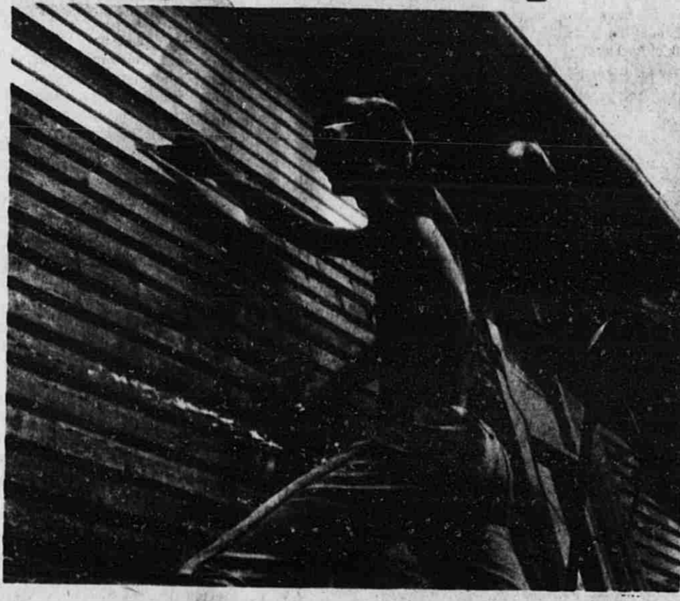
Both the pastors and parishioners have joined together to give St. Mary's Rectory on Lincoln Lake Avenue a badly needed facelift. This work to remove the old paint and apply a new coat is going ahead, while the study continues concerning whether to renovate or build a new church. Father Dick Lewis, right, and Semmarus Tom Page, are shown busy working on the rectory.
