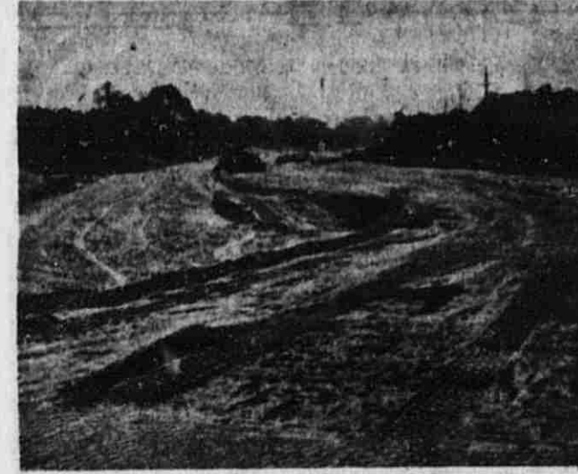
Crew spreads fill in the space from curb to blacktop bicycle path for the crew. The 108-year-old Old Collins School is in the far background.
