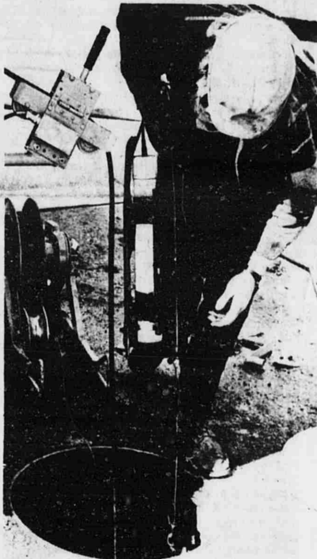
An A&B employee is shown here, lowering the closed circuit TV camera into a manhole. The camera will be pulled through the sewer line while an employee monitors the TV screen checking for leaks or breaks in the line. If a leak or break is seen, its exact location is noted for future reference when it is to be repaired.
