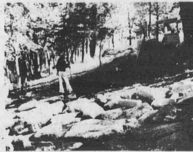
A front-end loader shoves pieces of concrete toward the crew at left. Finished riprapping is in the foreground.
