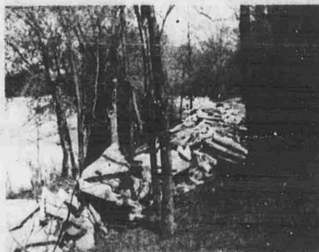
A 700-foot long row of concrete for riprapping has been placed on the banks of the Grand River at Ada's Chief Hazy Cloud Park.
