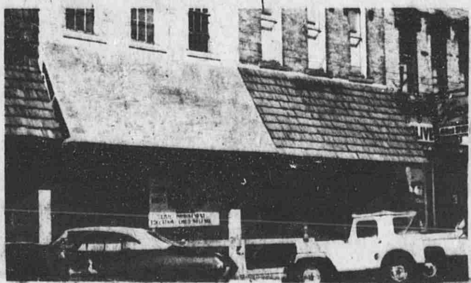
This view of the Saranac American Legion Post, shows the partially complete remodeling of the south building.
