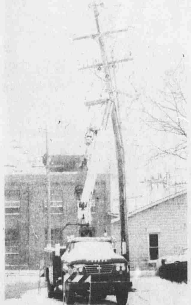
A circuit breaker pole by the Post Office was saved from completely toppling by the metal riser which acted as a brace. The pole, splintered midway was replaced.
